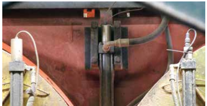
Cylinder position sensors installed in a lumber mill. Protective cap is missing from unit at right.
